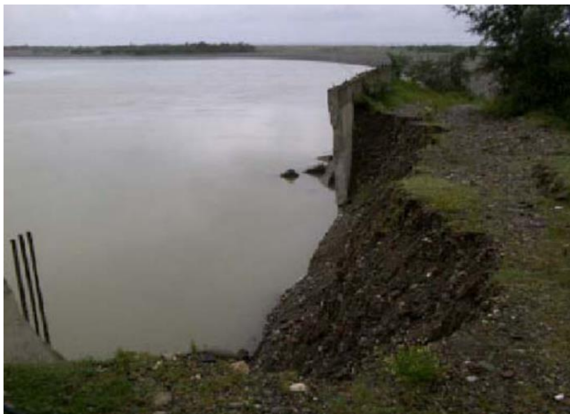
Fig. 3.16 Damaged protective wall in Batumi controlled waste disposal site
